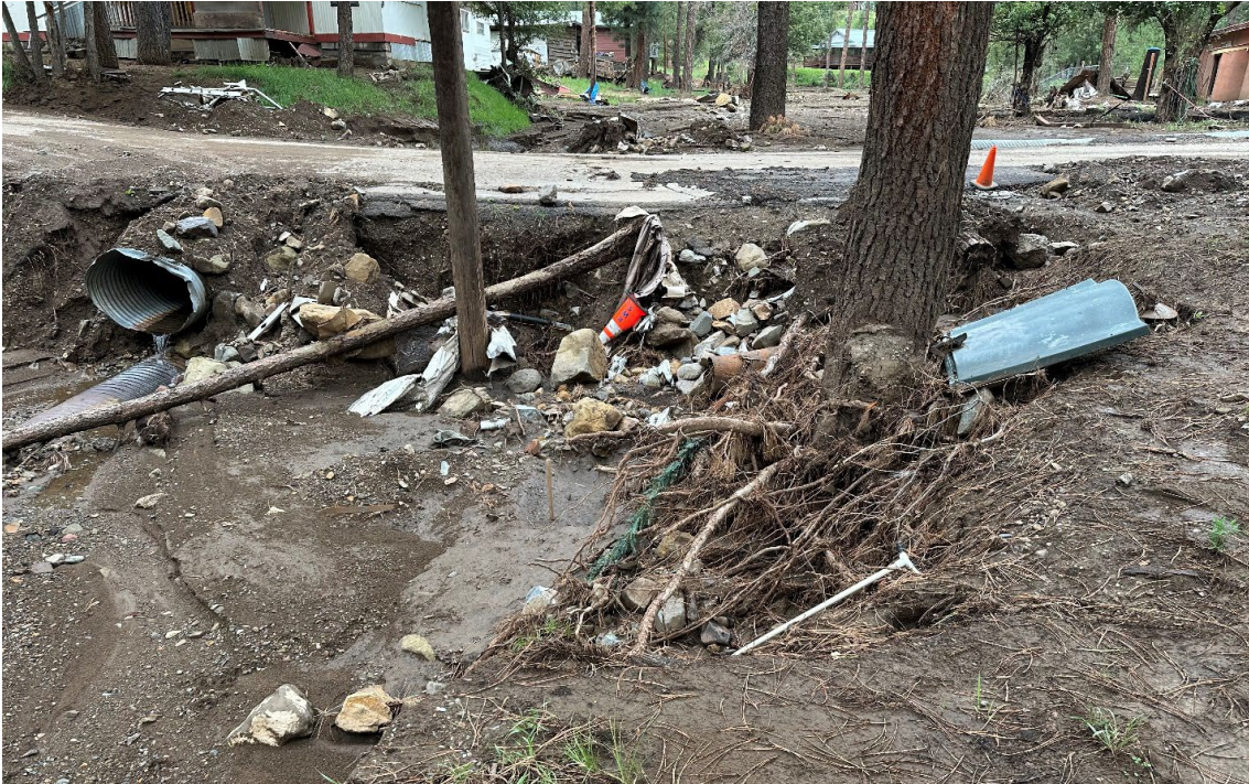
S. Oak Drive: Creek turned into a raging river causing extreme erosion and undermining roadways and depositing various types of debris.
