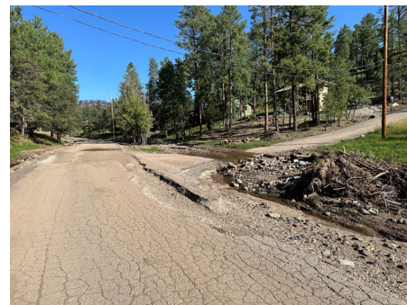
Perk Canyon Drive at Echo Drive: Post burn scarred watershed caused extreme flooding with heavy debris that filled the drainageways and caused the roadway to erode.
